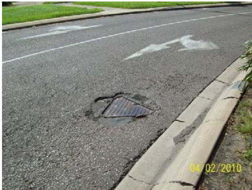
Manhole covers not matching road surface
