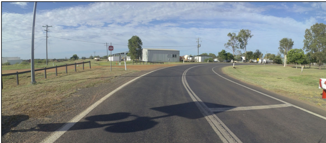
Photograph 6 – Capricorn Highway (just east of Lancewood Road – No Entry)
