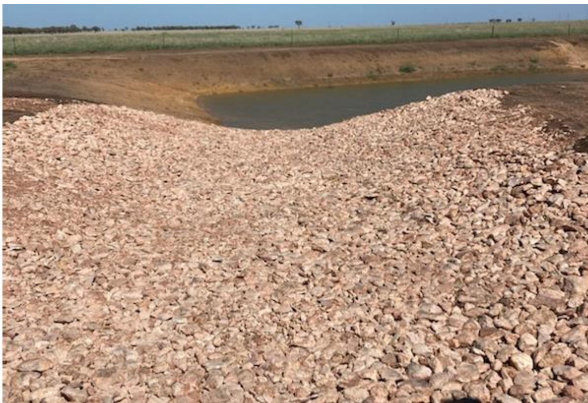
Figure 2: Photo showing rock lined channel inlet between stormwater drain and detention pond
