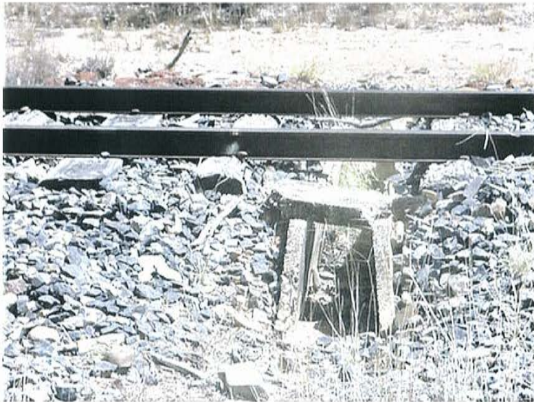
Plate 6 – Culvert in need of repair
