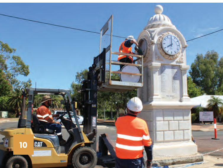
Below: Fixing the clock was also part of this year's capital works program.
