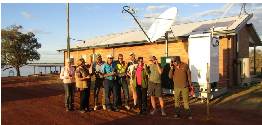
The Telstra 4G Mobile Satellite Small Cell tower being used by tourists at Lake Dunn.
